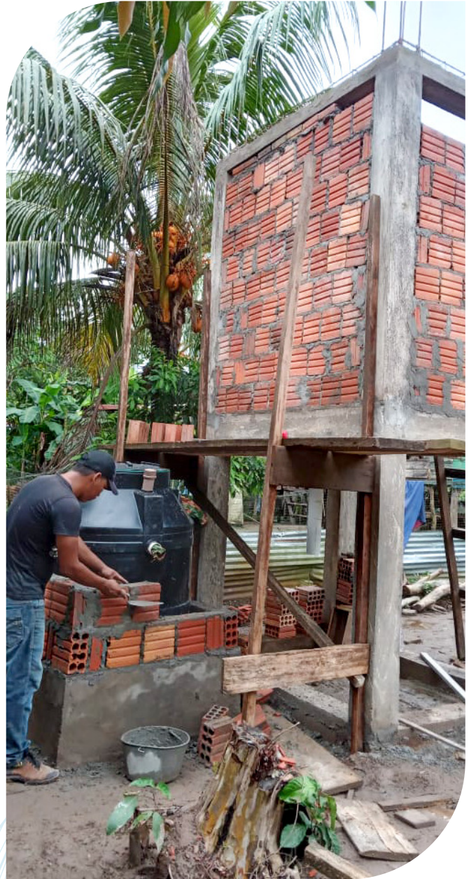
▲ WTW Amazon team works to complete the construction of a new community bathroom.
